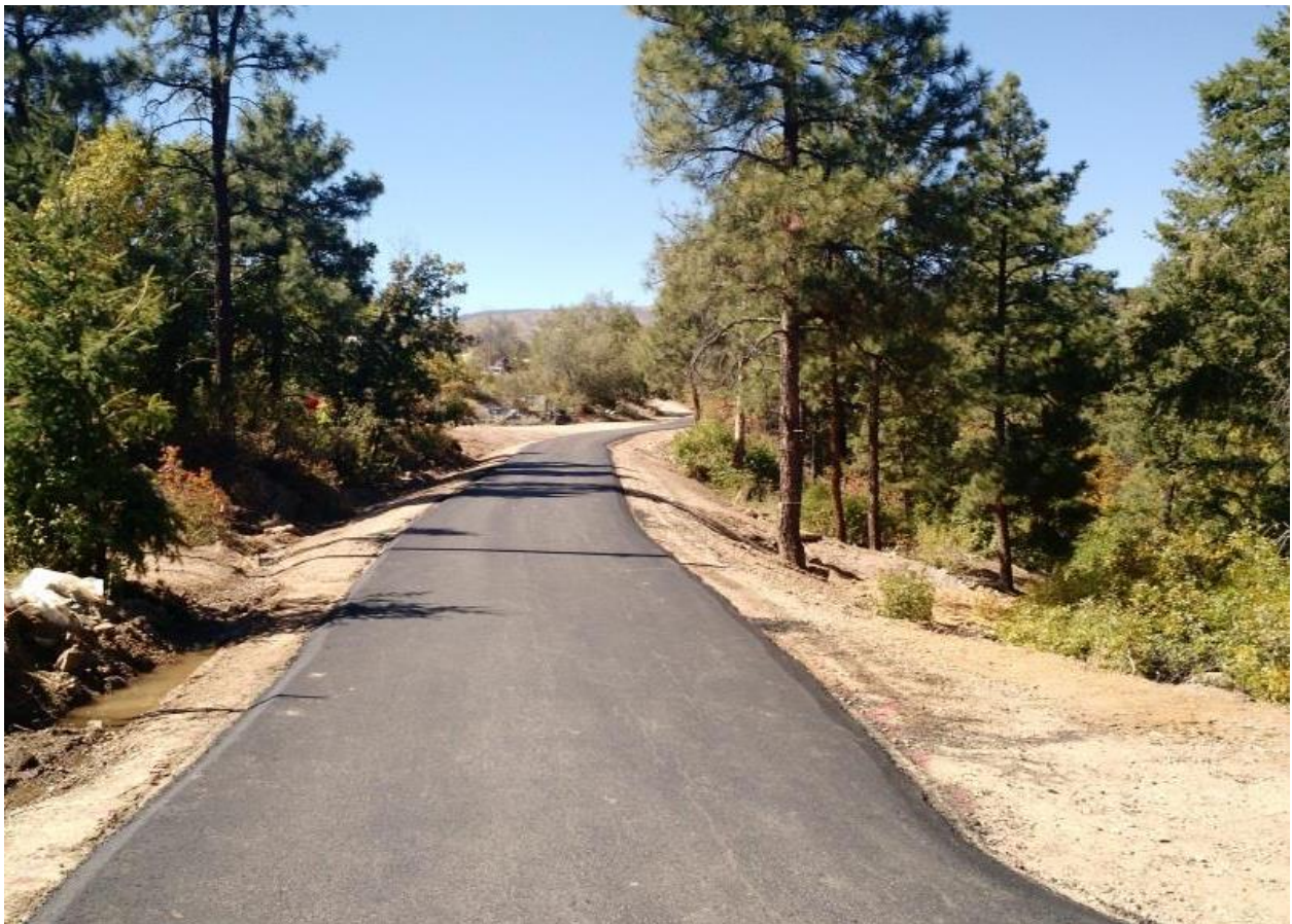
Above: Canyon Rim Multi-Use Path in Los Alamos; project received TAP funding in FFY14/15 and FFY16.
