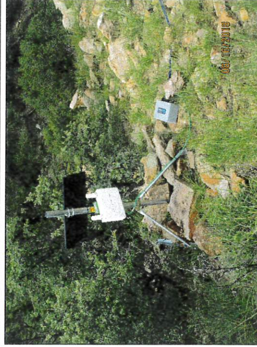
Photo 4: typical installation on I-25 at Romeroville (District 4) showing solar panel, cellular transmitter and data logger.
