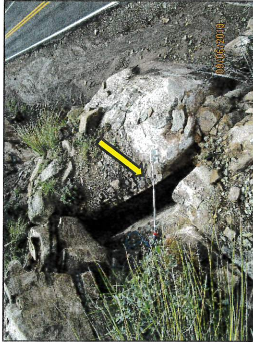
Photo 3: extensometer installed on NM 104 (District 4); sensor data shows progressive crack growth over the last year.
